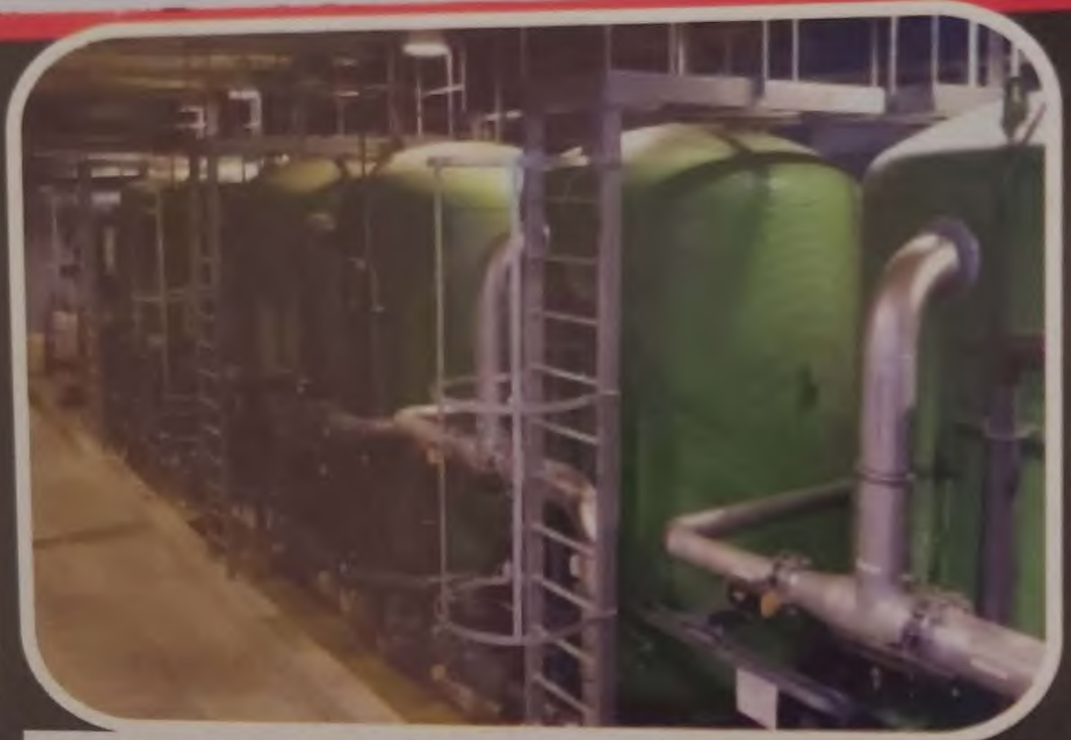
CONTROL : AIR TREATMENT/PURIFICATION
